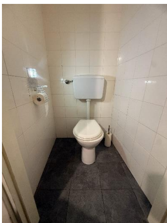
36 toilets without grab bars
